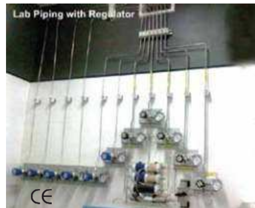
CE Lab Piping with Regulators
